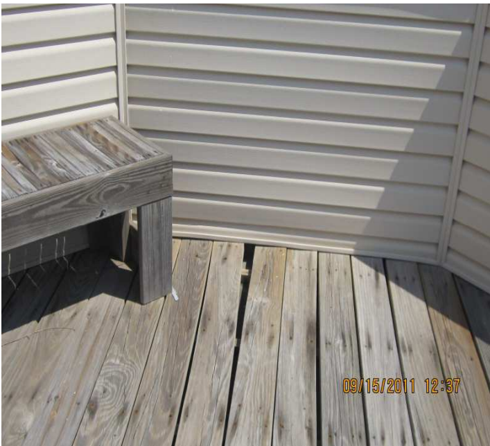
DAMAGED WOOD FLOORING AT CROWS NEST
