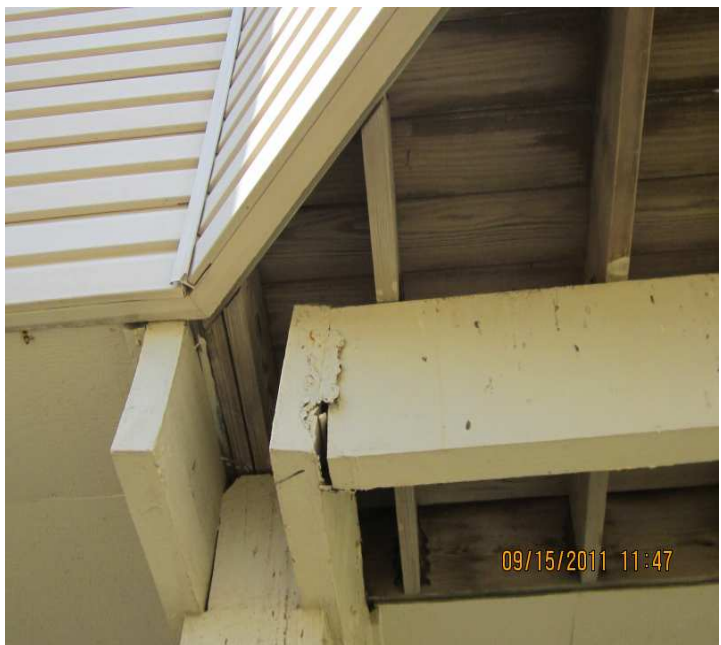
BACK CORNER OF HOUSE PULLING APART
