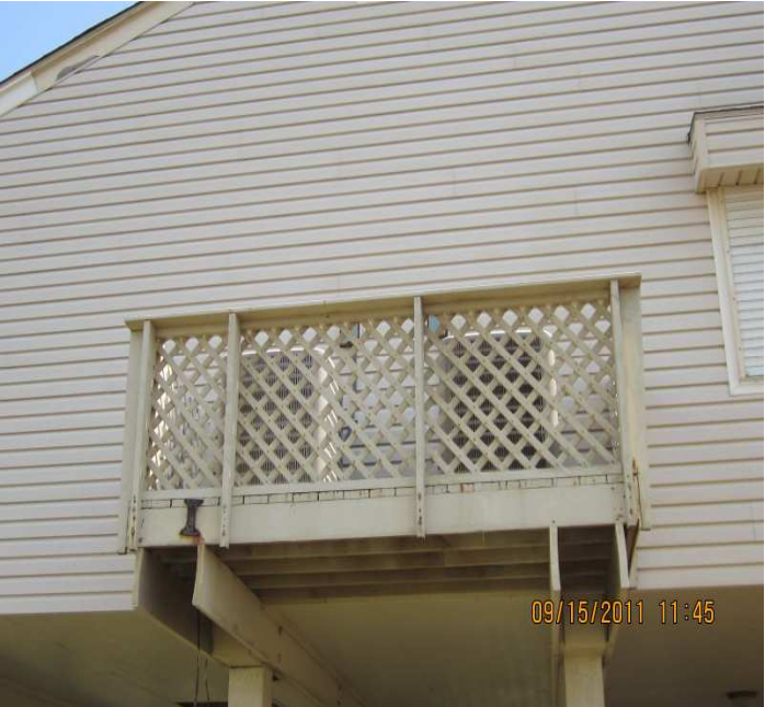
TWO A/C UNITS ON WEST SIDE PLATFORM
