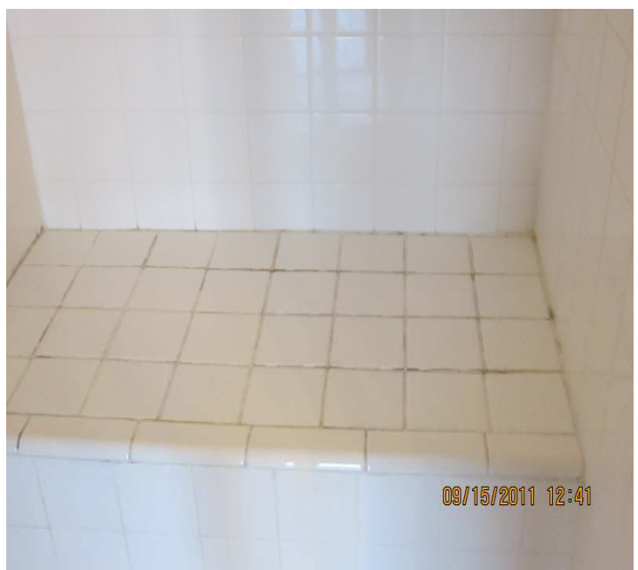
DAMAGED CERAMIC TILE & BENCH IN BATH SHOWER
