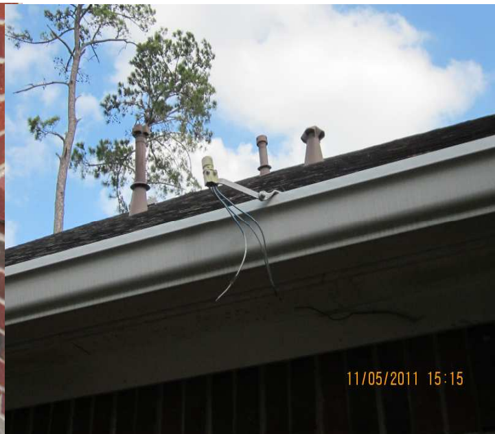
DAMAGED RAIN GAUGE ON WEST EAVE
