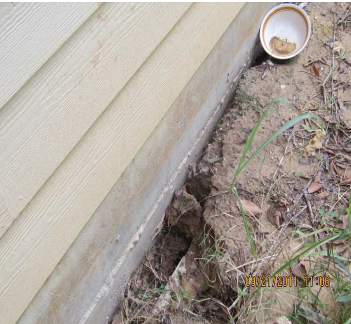
GAPS, N GROUND, BY BACK SIDE SLAB
