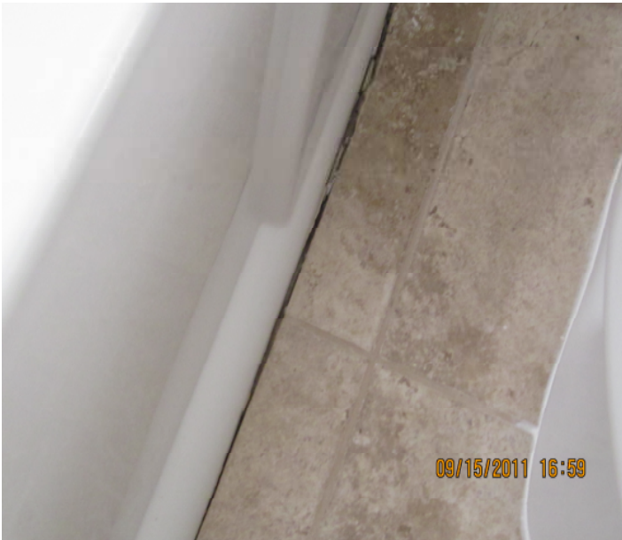
GAPS BETWEEN TUB AND FLOOR TILE IN # 2 BATH
