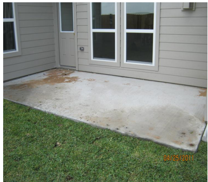
BACK PATIO NEEDS TO BE SCRAPED & WASHED DOWN
