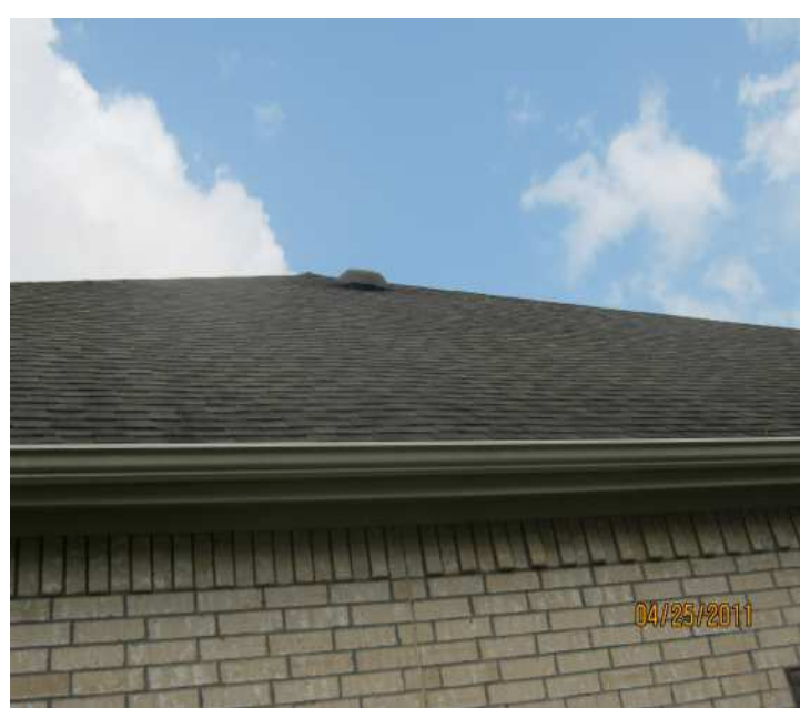
DAMAGED ROOF SHINGLES ON SOUTH SIDE
