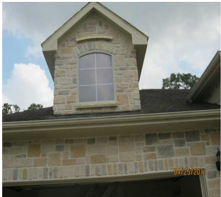
DAMAGED METAL ROOF FLASHING LOWER FRONT ROOF
