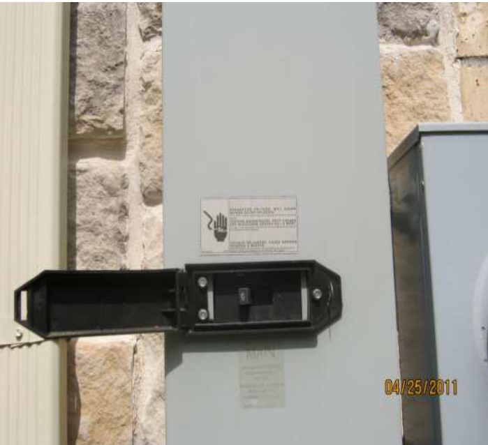
MAIN BREAKER BOX ON OUTSIDE SOUTH WALL
